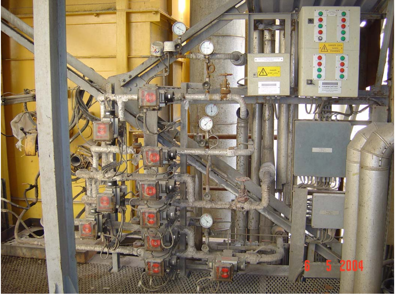
SODA SANAYİİ A.Ş. – 4 adet DF-815 Brülör, fuel-oil vana grubu
